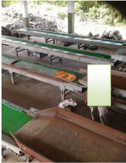
Figure 4.2: Conveyor Belts used for Waste Separation
